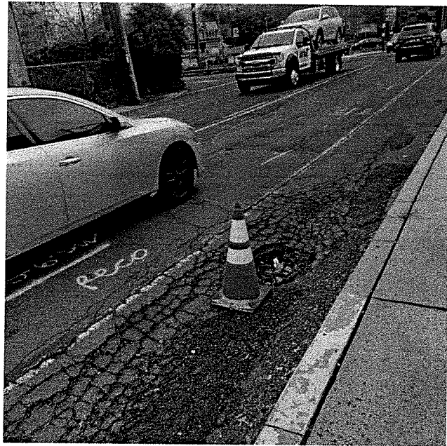
Hole Before Repair
